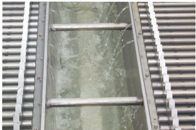
Phase I: Clarification facility. clarified water
